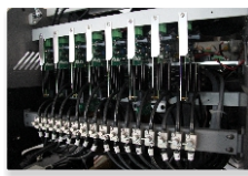
Negative Pressure System
